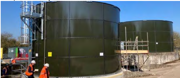
A typical set of storm tanks as installed at Fakenham.
